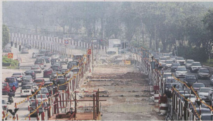
The ongoing LRT construction along Jalan Langat will benefit Klang's residents as it will improve the overall infrastructure in the municipality.
